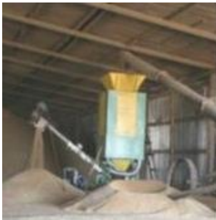
Figure 1.2. Microwave installation “AST-3”
